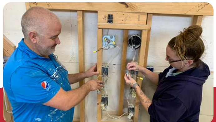
Bill Lewis, Clearview School Career Technical Instructor working with the Construction Trades Apprentice on the grounds of the Ohio Reformatory for Women (ORW).
